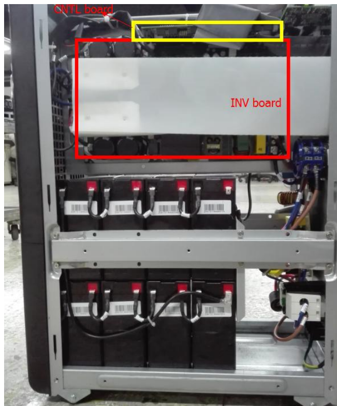
Fig. 4.4.3 Boards in 6K Tower
